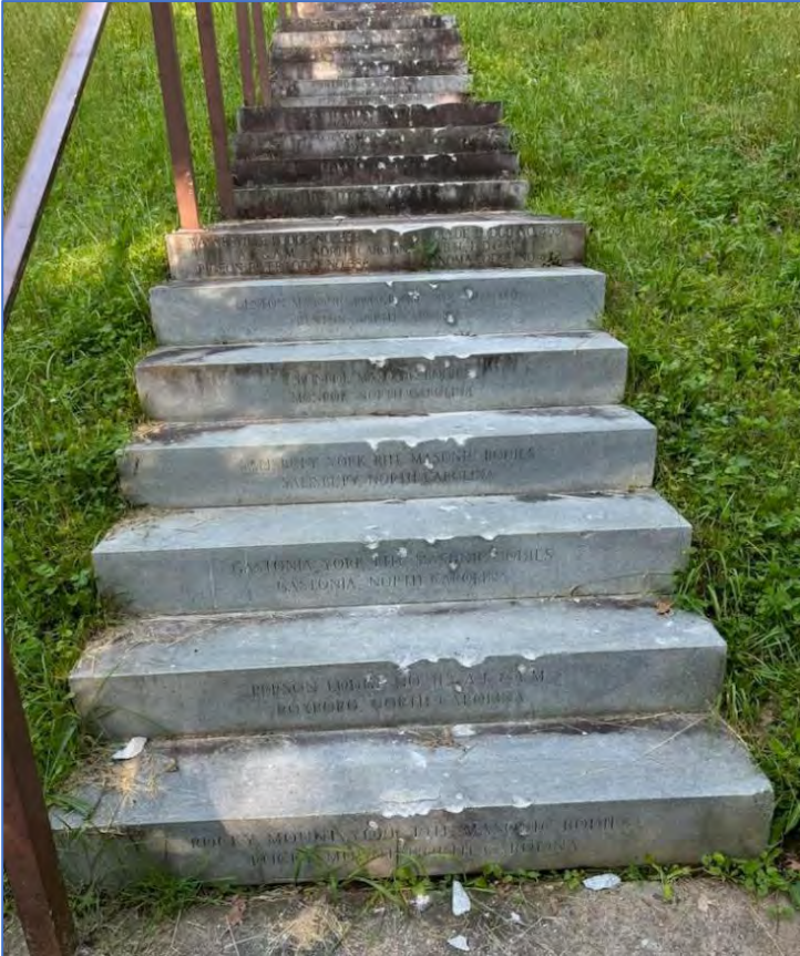
The steps on the staircase leading up the hill to the marker were also damaged. The repairs to the marker and surrounding structures will be very expensive and will take months to complete.
